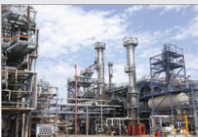
Refinery equipment (option)
